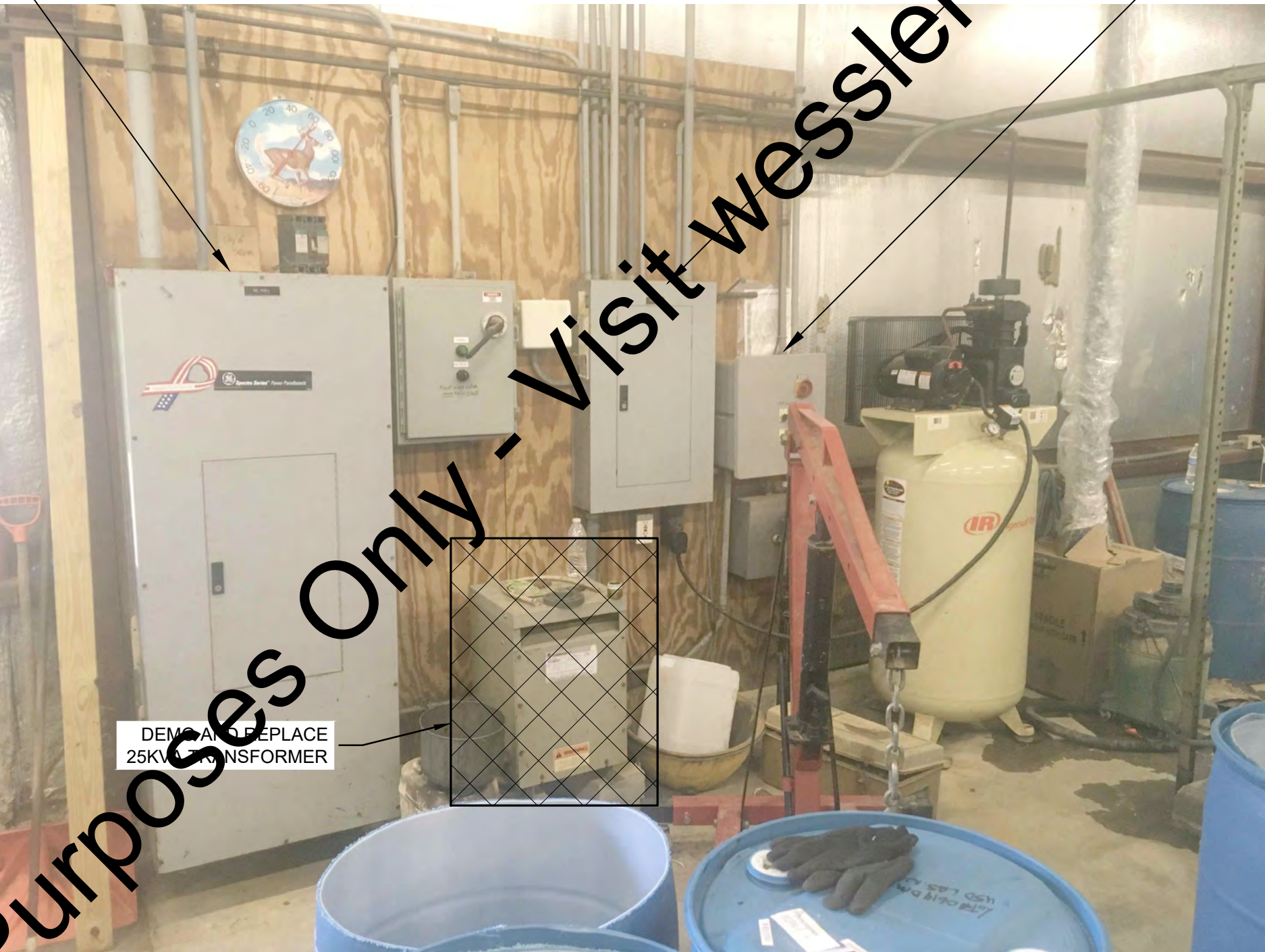
EX POWER PANEL, PLANT WASH CONTROL PANEL, TRANSFORMER AND LIGHTING PANEL
