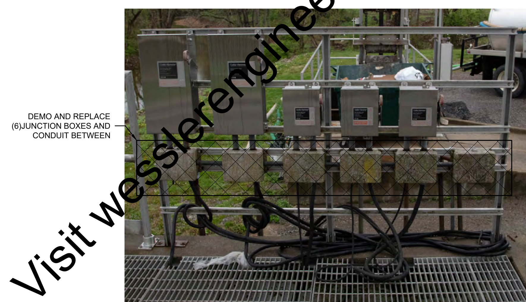
EXISTING RAW SEWAGE PUMP DISCONNECTS AND JUNCTION BOXES
