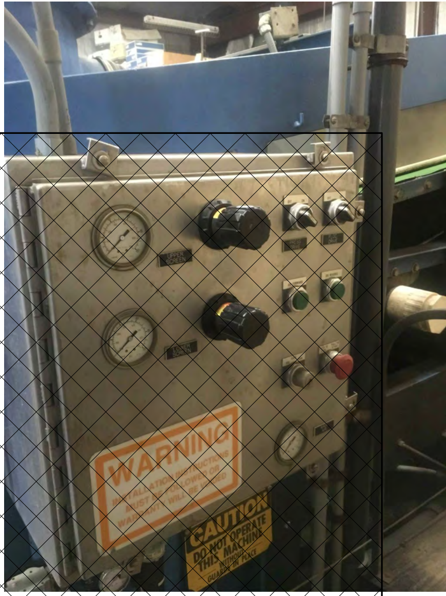
EX BELT PRESS CONTROL PANEL
