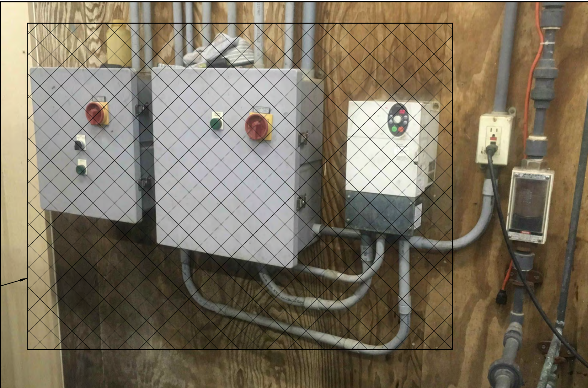
EX AUGER CONTROL PANEL, EX BELT PRESS POWER JUNCTION BOX, AND SLUDGE PUMP VFD
