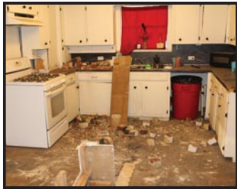
Damage to the Epsilon Tau kitchen
