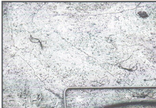
Thermal cracks in a thick slab
