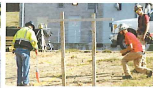
The ceremonial groundbreaking for the City of Salem's $15.2 million water plant project was held against a backdrop of bustling activity. Heavy equipment operators were moving earth and workers were marking the ground while officials lauded the project to update the aged facility.
