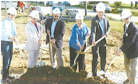
A symbolic groundbreaking ceremony was held Monday for the project. Shown from left are Congressman Troy Hollingsworth, Salem Mayor Troy Merry, Salem Common Council President Justin Green, Salem Clerk-Treasurer Sally Hattabaugh, Indiana Bond Bank Executive Director Mark Wuellner, and USDA Rural Development Community Programs Southern District Director Craig McGowan.
