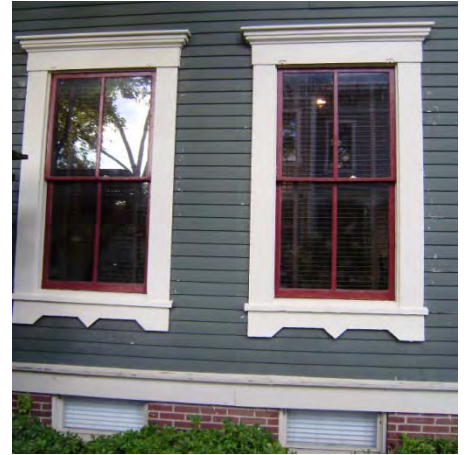
Bi-glass system of double thickness replacement glass in historic window
